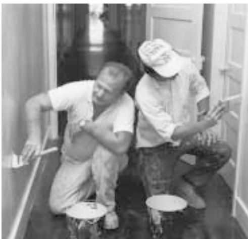
Members of the community pitched in and helped spruce up the facility
